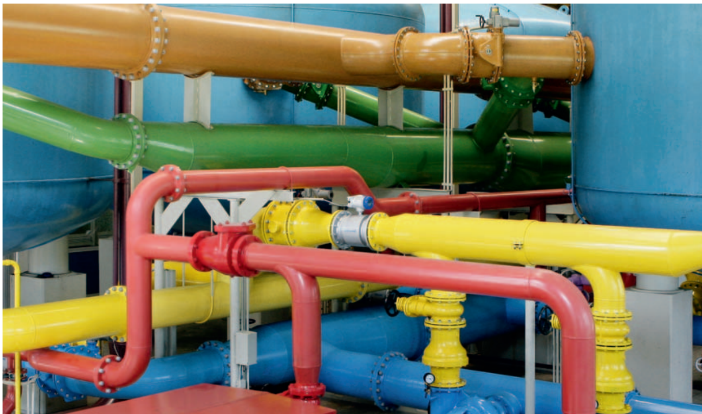
OPTIFLUX 4300 in the filtration system in the Haltern waterworks
